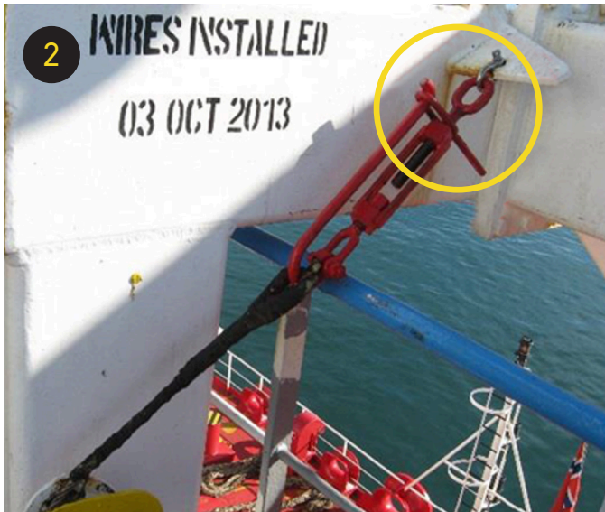
FIGURE 2 THE TURNBUCKLE AND THE PIN MARKED WITH A YELLOW CIRCLE) AFTER THE MAINTENANCE JOB HAD BEEN CARRIED OUT. SOURCE: AIBN; USCG
