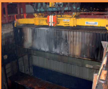
Heat damage and smoke staining to container and the hold caused by a charcoal fire.
