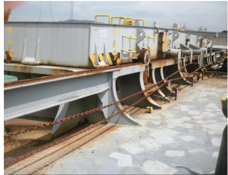
Poorly adjusted drive chains
