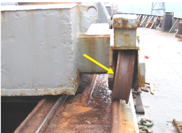
FIGURE 3 Hatch cover guide wheel bearing failed - hatch cover will not close evenly
