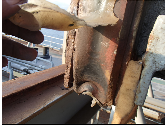
FIGURE 9 Silicone applied in an attempt to effect proper sealing
