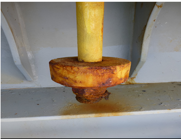
FIGURE 10 Hatch securing cleat, seized and painted over
