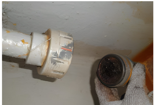
FIGURE 2 Hatch coaming drain completely blocked with debris and rust
