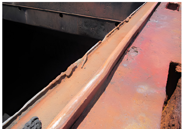
FIGURE 4 Mechanical damage to the compression bar and inner drain channel
