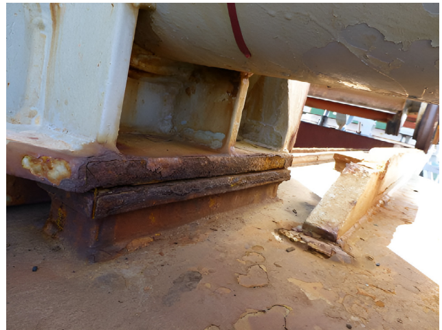
FIGURE 5 Corroded and wasted hatch cover landing pads
