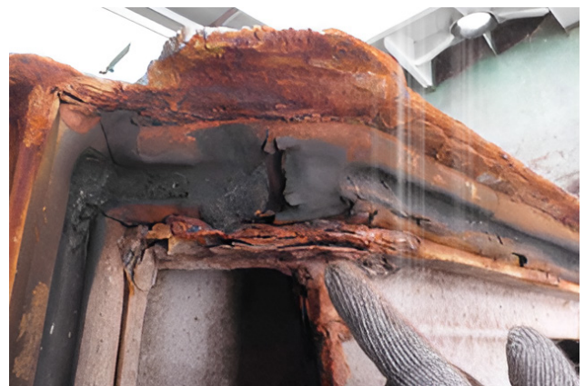
FIGURE 8 Hatch cover sealing rubbers damaged and showing permanent deformation beyond the recommended limits. Rubber seal channels severely corroded.
