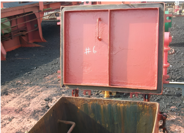
FIGURE 6 Evidence of water ingress at the cargo hold entrance hatch and the hatch coaming
