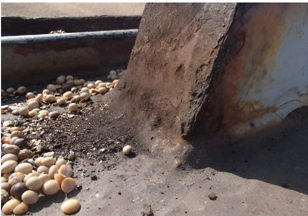
FIGURE 1 Hatch coaming not swept, cargo debris and rust still evident. Centreline joint closing wedge showing severe wear
