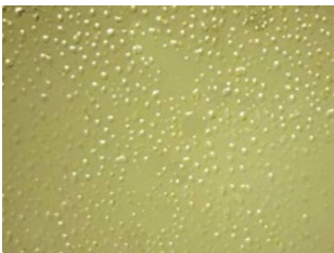
Unbroken coating blister
