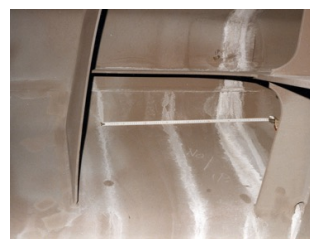
Damaged coating (Zinc salt)
